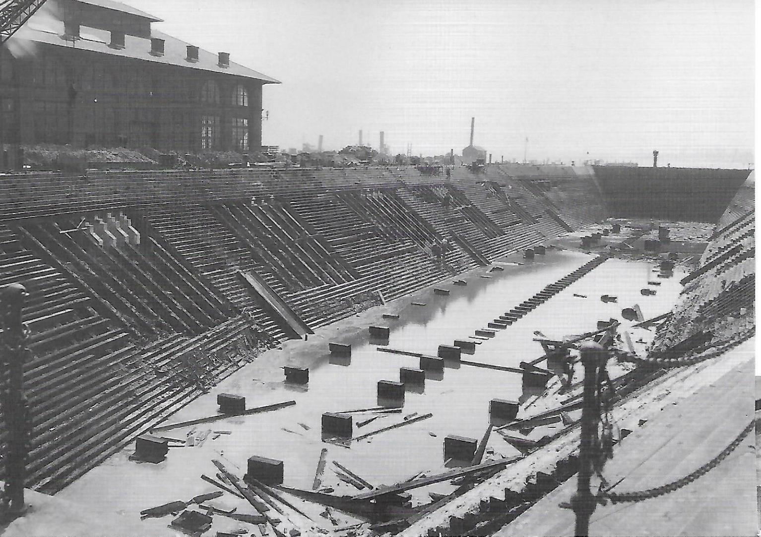
Dry Dock No. 1, 1928. Built in 1891, it leaked so badly during the 1920s that it could not dock ships. Commandant Thomas P. Magruder's persistent request for repair contributed to his removal from command. NARA Washington, D.C., Still Picture Branch.
